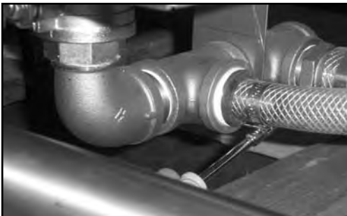
Loosening the rinse drain hose from the rinse drain nipple
