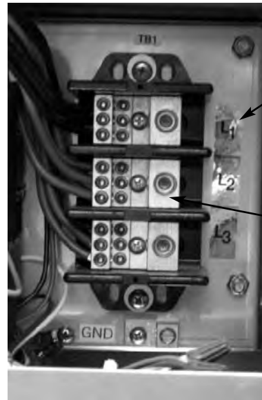
Incoming Power Connection
